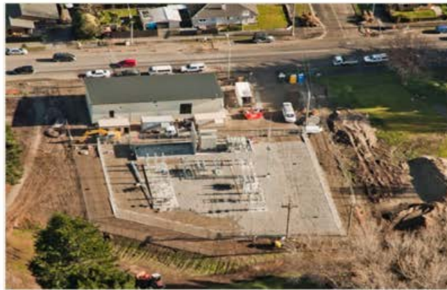
Figure 28: Replacement Zone Substation
