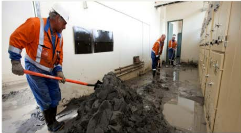
Figure 18: Liquefaction Inside Major Substation
