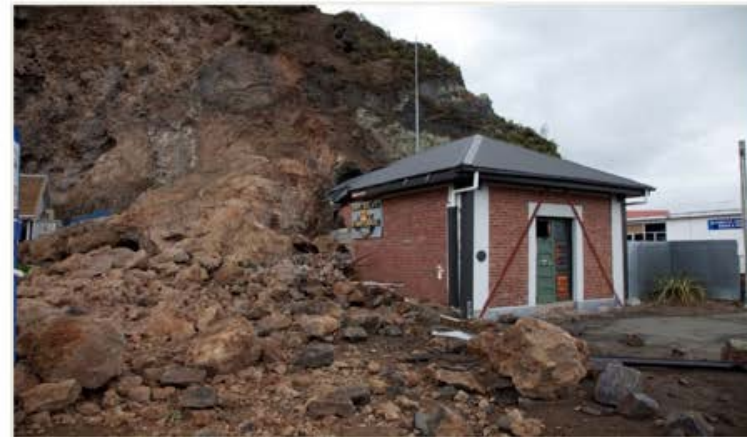
Figure 21: Substation Rock Fall Damage
