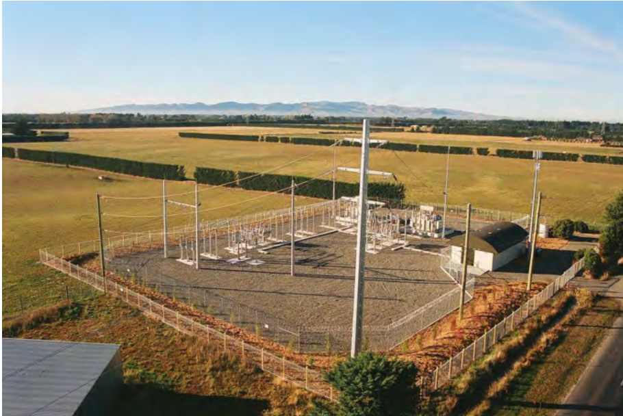
Weedons 66kV rural zone substation
