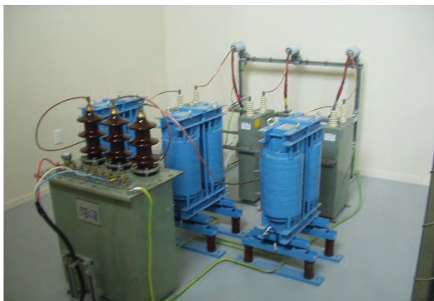
11kV injection plant at a zone substation.
