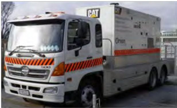
Mobile generator truck
