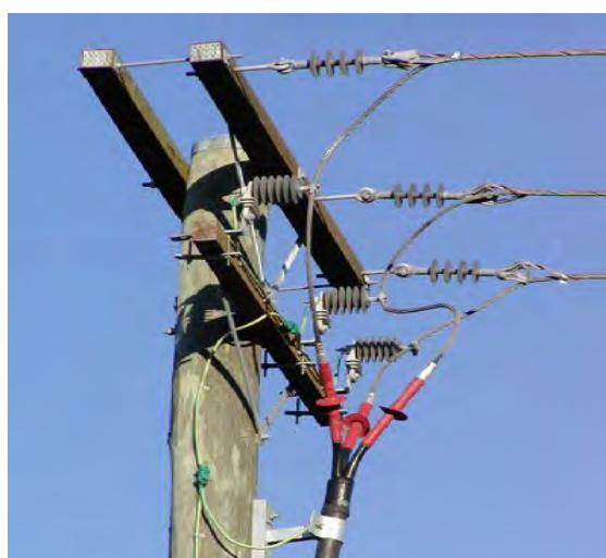
Overhead line 11kV cable termination with surge arrestors fitted
