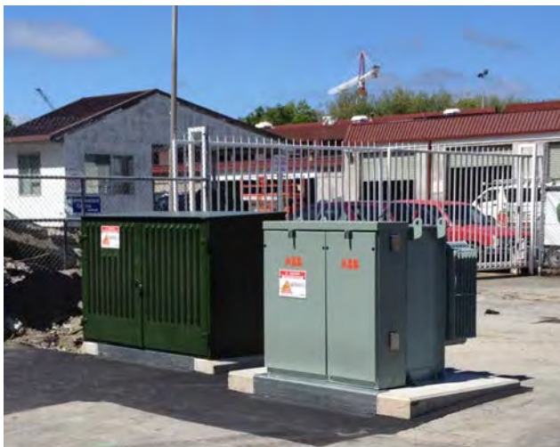
Outdoor substation - consisting of a half-kiosk and adjacent transformer.
