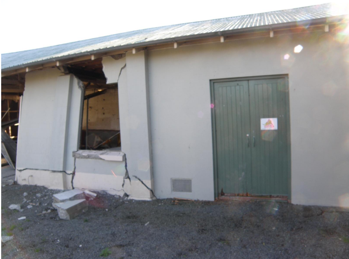
Figure 9: Redcliffs waterworks substation
